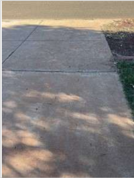
Exterior 02/05/2023 3:53 PM Image 441 :Driveway
