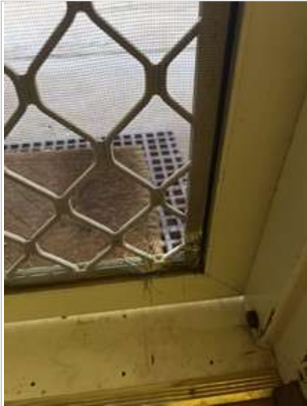
Dining Room 02/05/2023 3:45 PM Image 347 :Door/ Doorframe
