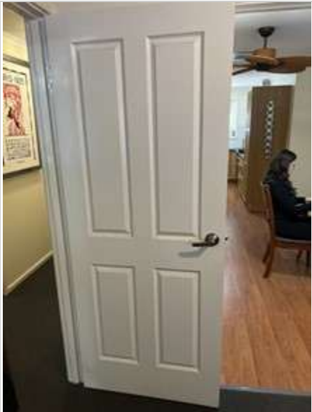
Lounge Room 02/05/2023 2:24 PM Image 122 :Door/ Doorframe
