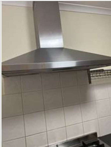
Kitchen 02/05/2023 2:59 PM Image 311 :Exhaust Fan/ Rangeh..
