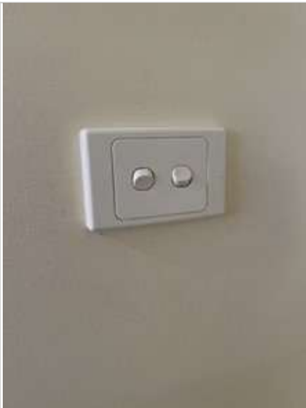
Bathroom 02/05/2023 1:57 PM Image 192 :Lights/ Fixtures
