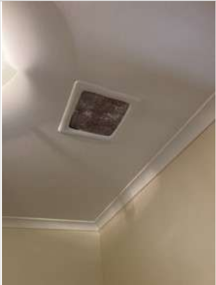
Laundry 02/05/2023 2:02 PM Image 396 :Exhaust Fan/ Vent
