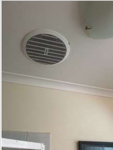
Bathroom 02/05/2023 1:57 PM Image 193 :Exhaust Fan/ Vents
