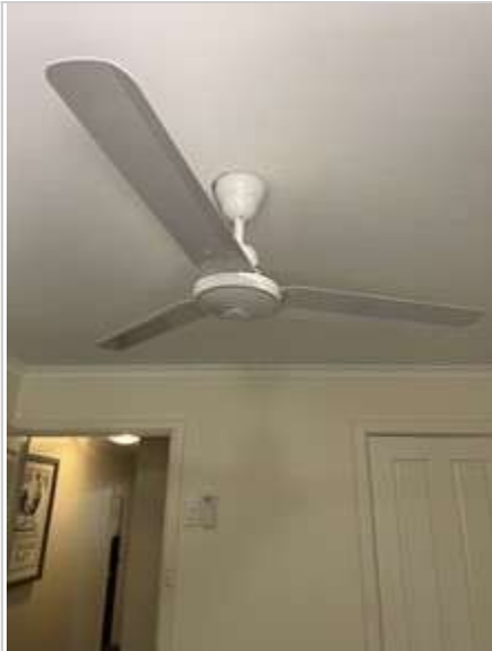
Bedroom 2 02/05/2023 2:15 PM Image 257 :Lights/ Fixtures
