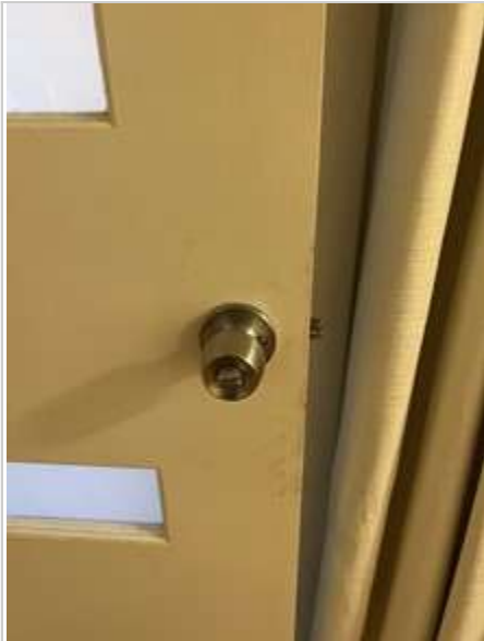
Dining Room 02/05/2023 3:45 PM Image 345 :Door/ Doorframe
