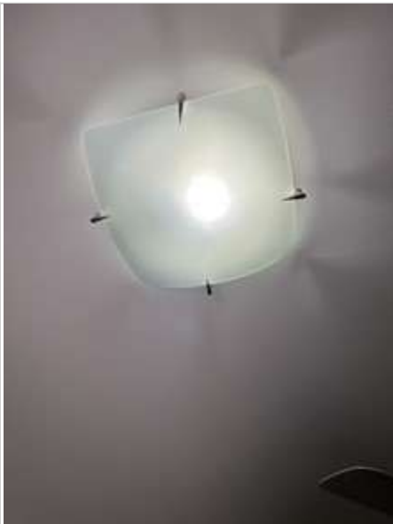
Bedroom 2 02/05/2023 2:15 PM Image 256 :Lights/ Fixtures
