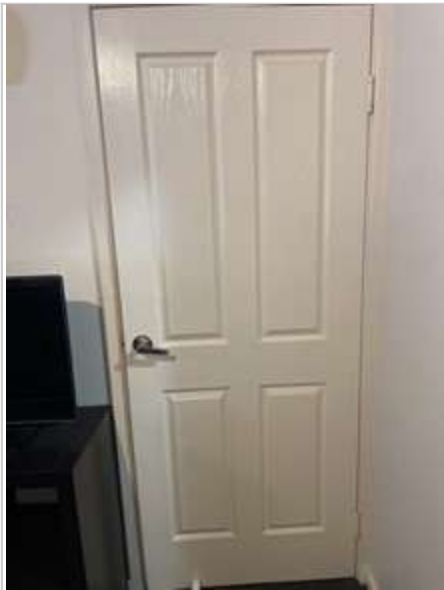
Lounge Room 02/05/2023 2:24 PM Image 123 :Door/ Doorframe
