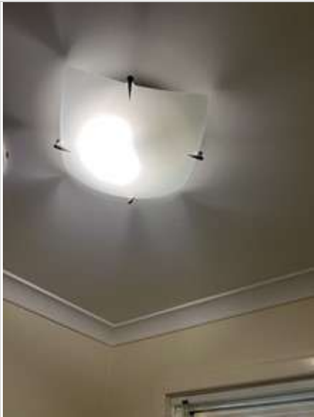
Bathroom 02/05/2023 1:57 PM Image 190 :Lights/ Fixtures
