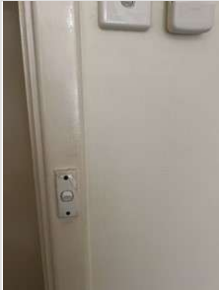
Bedroom 2 02/05/2023 2:19 PM Image 259 :Lights/ Fixtures
