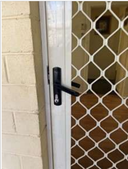
Dining Room 02/05/2023 3:45 PM Image 351 :Door/ Doorframe
