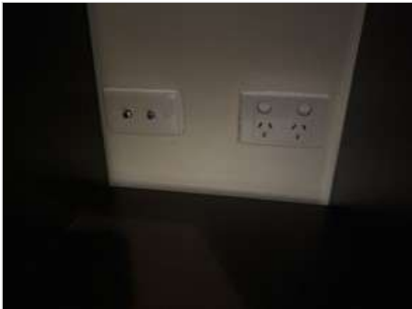
Lounge Room 02/05/2023 2:24 PM Image 124 :Powerpoints/ Fixt...
