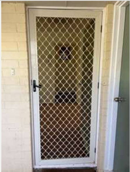
Dining Room 02/05/2023 3:45 PM Image 350 :Door/ Doorframe
