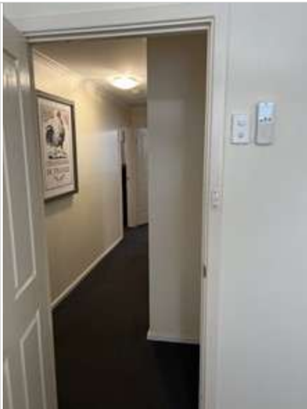
Bedroom 2 02/05/2023 2:14 PM Image 248 :Door/ Doorframe
