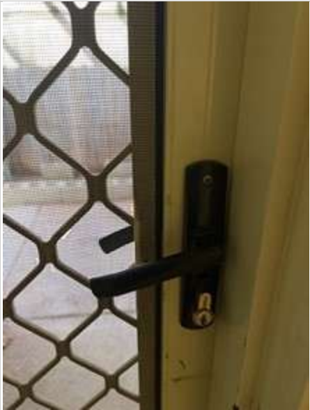
Dining Room 02/05/2023 3:45 PM Image 348 :Door/ Doorframe
