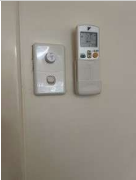
Bedroom 2 02/05/2023 2:19 PM Image 258 :Lights/ Fixtures
