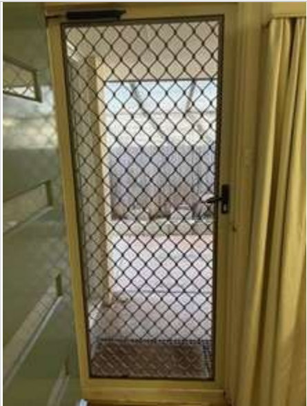
Dining Room 02/05/2023 3:45 PM Image 346 :Door/ Doorframe
