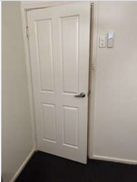
Bedroom 2 02/05/2023 2:13 PM Image 246 :Door/ Doorframe
