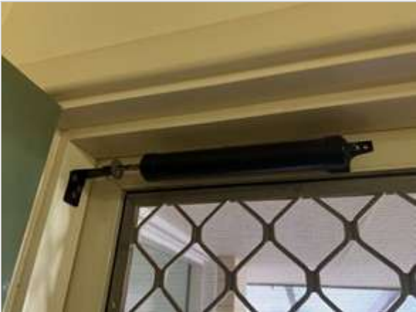
Dining Room 02/05/2023 3:45 PM Image 349 :Door/ Doorframe
