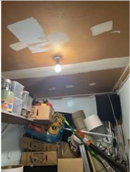
Storeroom 02/05/2023 3:08 PM Image 520 :Lights/ Fixtures
