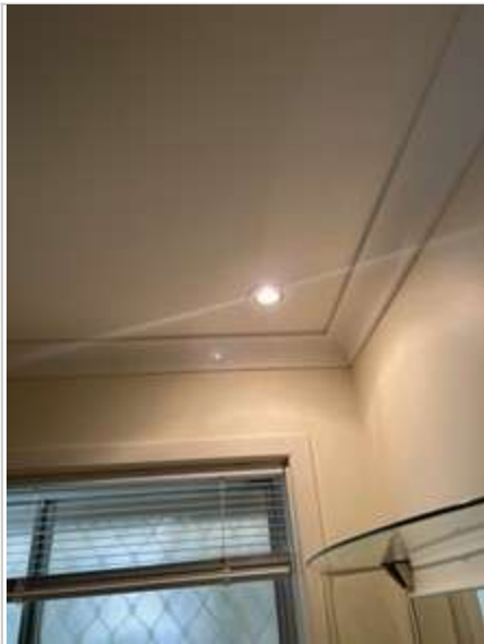
Bathroom 02/05/2023 1:57 PM Image 191 :Lights/ Fixtures
