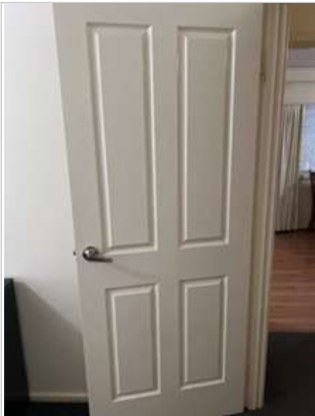
Bedroom 2 02/05/2023 2:13 PM Image 247 :Door/ Doorframe
