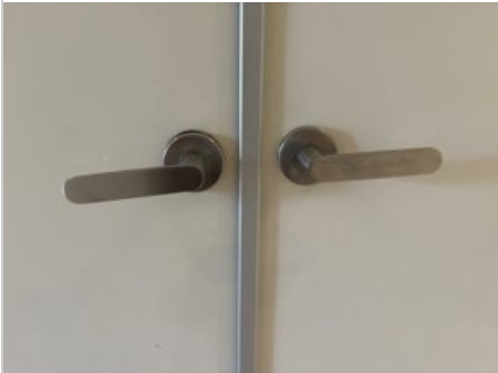
Family room 17/03/2025 2:13 PM Image 447 :Door/ Doorframe
