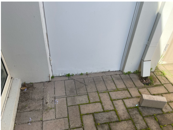
Deterioration noted to the garage rear door. This common with external doors. Recommend repair/treat and paint
