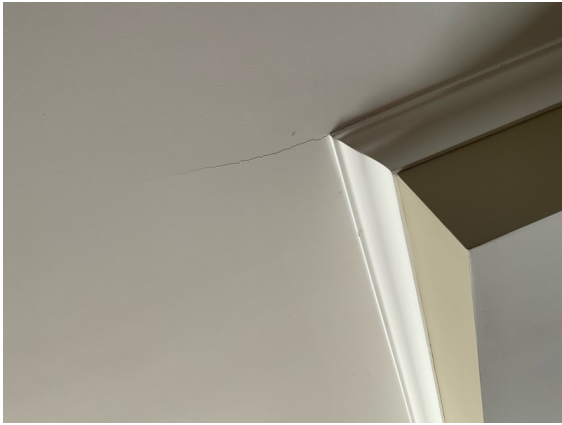
Minor appearance ceiling crack noted to the kitchen ceiling at the bulkhead. This is common with bulkhead ceilings at corners. Recommend repair and paint.
