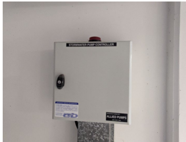
9.02 Stormwater pump controller
