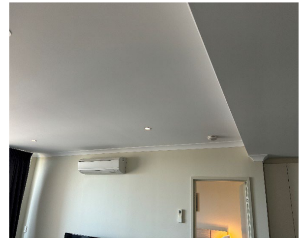
Smoke detection within units
