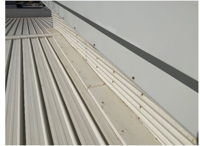
2.03 Corrosion to fasteners
