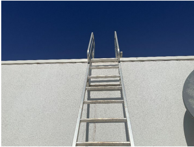
2.04 Roof access equipment
