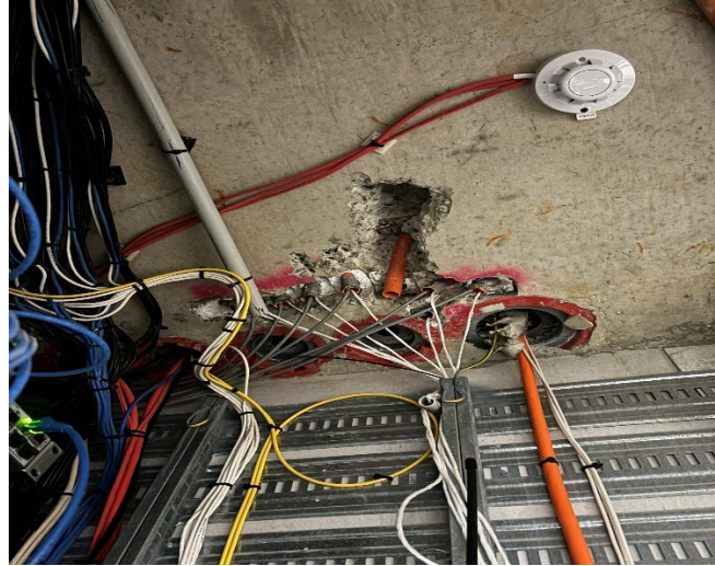
Poorly protected services penetrations – DB enclosure
