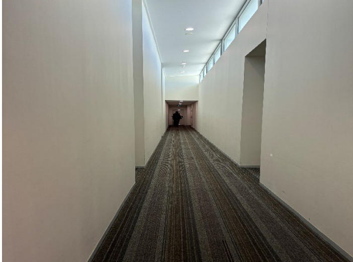
Corridor exceeds 40m – no smoke separation
