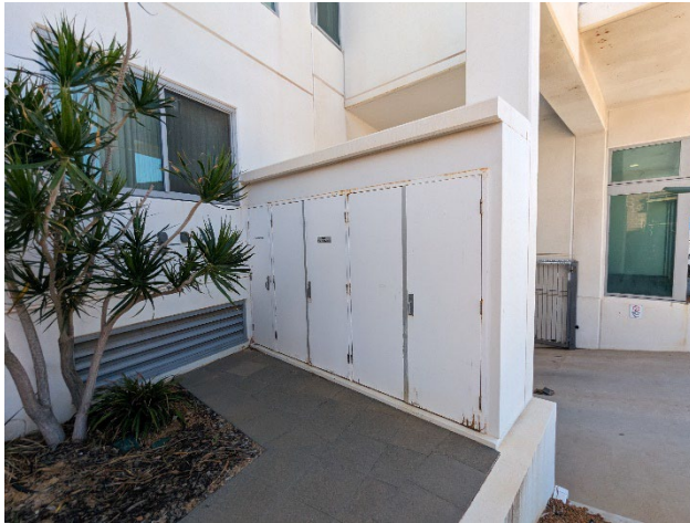
7.01 Site main switchboard
