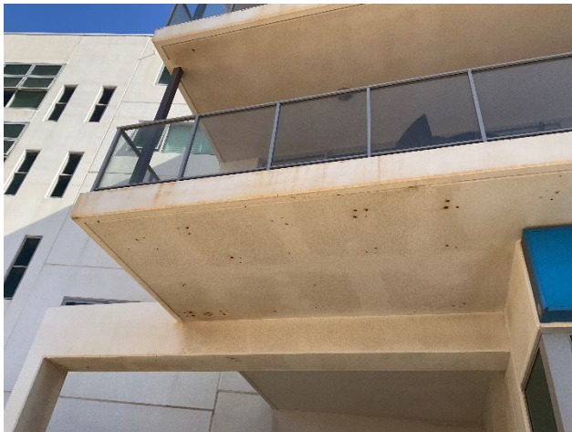
3.06 The external façade is demonstrating signs of paint and render deterioration.
