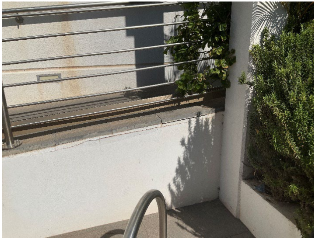
3.03 Waterproofing to planter boxes typically has a design life of 10 -15 years.
