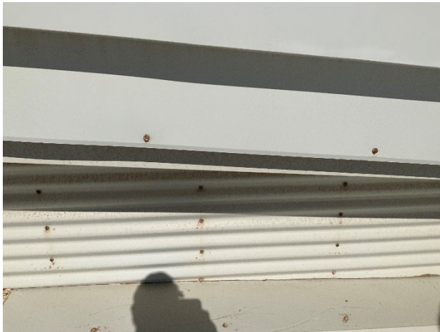
2.03 Corrosion to fasteners
