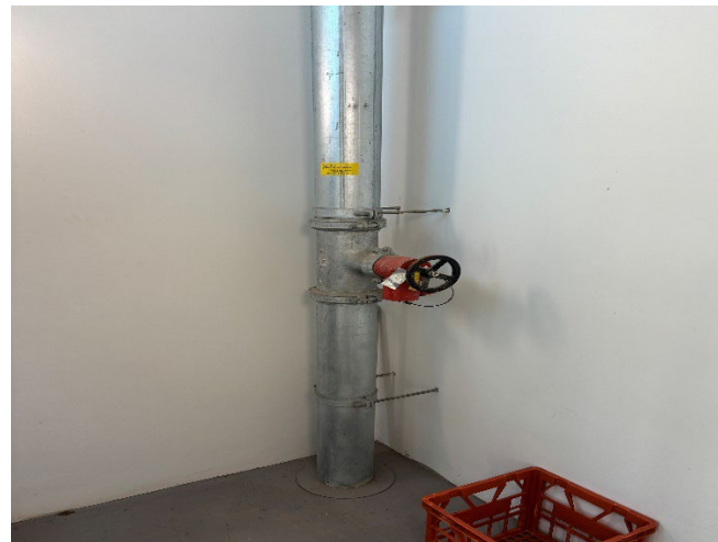
Internal hydrants within fire-stair
