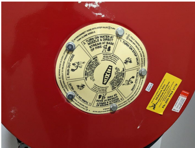
8.02 Fire hose reel
