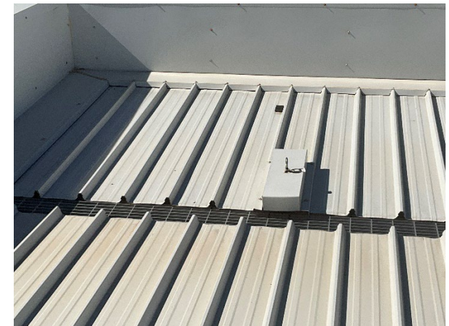
2.04 Roof access equipment
