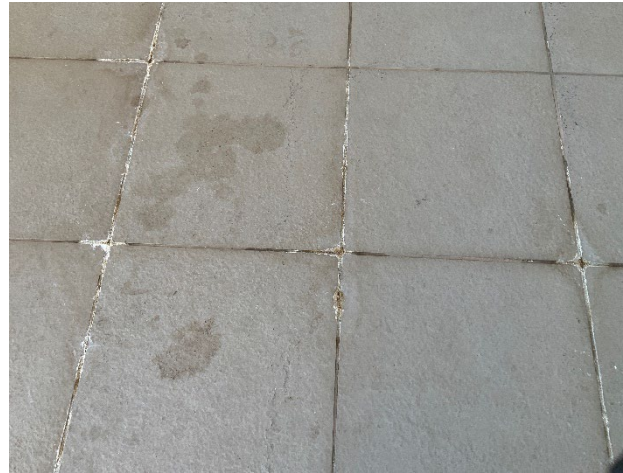
1.03 Calcium deposits and chalky residue to tiled grout lines
