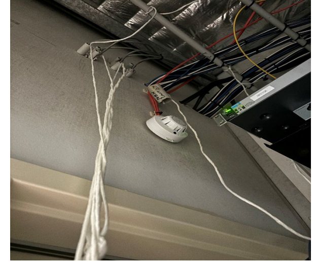
Poorly protected services penetrations & Wall mounted smoke detector
