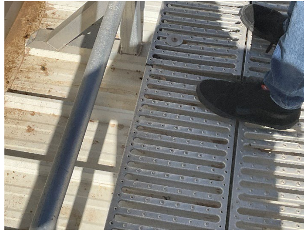
2.04 Roof access equipment
