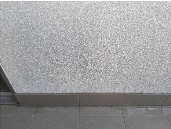
Fiore Apartments – Unit 5 Balcony: Close-up view of the silicone seal applied to the grout joint and the bubbling render finish.
