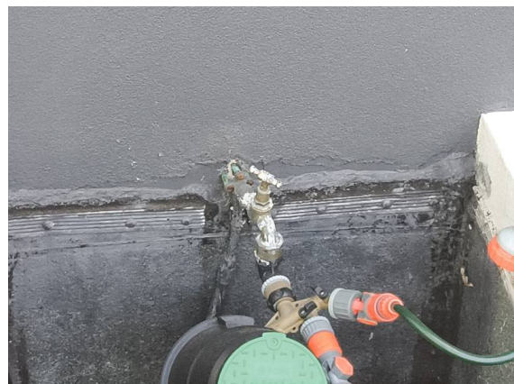
Fiore Apartments – Unit 5 Balcony: Adjoining balcony directly behind Bed 1 of Unit 5. Close up displaying where tap has come off wall leaving holes for potential moisture ingress.
