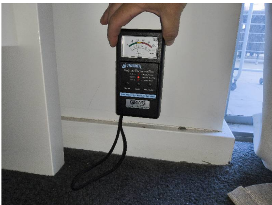
Fiore Apartments – Bedroom 2: A control moisture reading was taken in close proximity to the affected area on a section of wall that showed no signs of moisture. This reading measured 14 percent.
