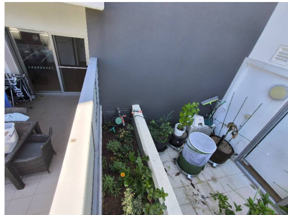
Fiore Apartments – Unit 5 Balcony: The adjoining balcony located directly behind Bedroom 1 of Unit 5 shows standing water on the floor despite there being no rainfall for more than 10 days, indicating the moisture is likely originating from the reticulation system.
