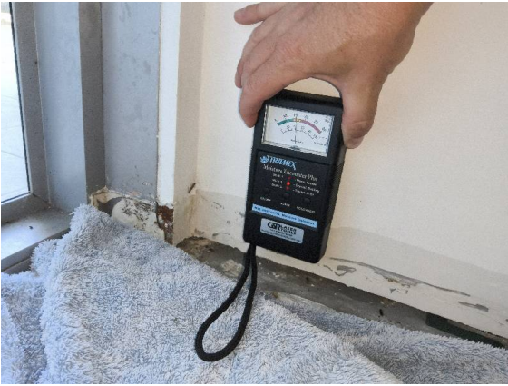
Fiore Apartments – Bedroom 2: A moisture reading taken closer to the planter box recorded 16 percent.
