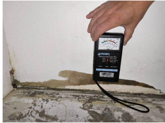
Fiore Apartments - Bedroom #1: Moisture readings exceeding the measurable range of the moisture meter.
