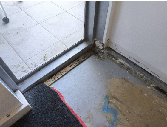
Fiore Apartments – Bedroom 2: View of affected areas.
