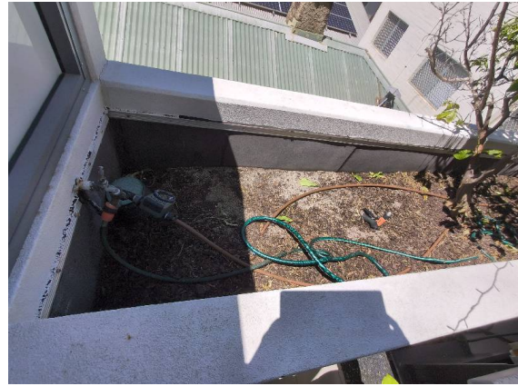
Fiore Apartments – Unit 5 Balcony: Unit 5 balcony planter, tap and reticulation - no signs of damage or moisture present.
