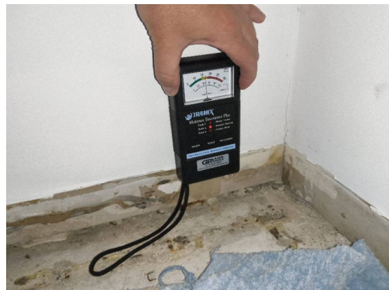
Fiore Apartments – Bedroom 2: A moisture reading taken closer to the planter box recorded 18 percent.
