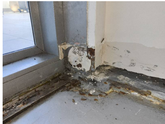
Fiore Apartments – Bedroom 2: View of affected areas with visible rust to corner beads and carpet trims.
