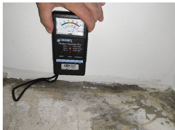
Fiore Apartments - Bedroom #1: Lowest moisture reading taken at 25%.
