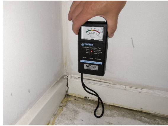
Fiore Apartments – Bedroom 2: A moisture reading taken closer to the robe recorded 10 percent.
