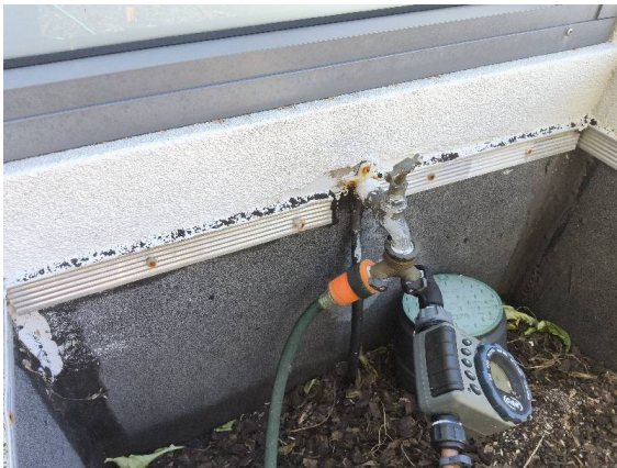
Fiore Apartments – Unit 5 Balcony: Unit 5 balcony planter, tap and reticulation. Recommend to replace screws with more suitable non-rusting and silicone seal.
