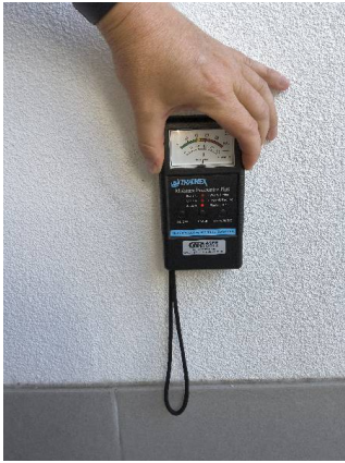
Fiore Apartments – Unit 5 Balcony: Moisture reading taken next to bubbling render finish measuring 25%.
