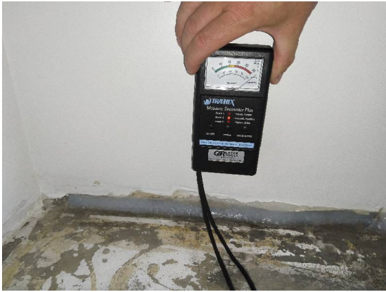
Fiore Apartments - Bedroom #1: Moisture readings exceeding the measurable range of the moisture meter.
