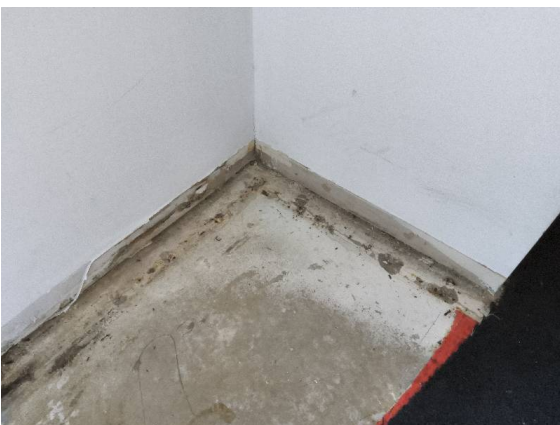
Fiore Apartments – Bedroom 2: View of external corner of robe with visible rust to steel studwork.
