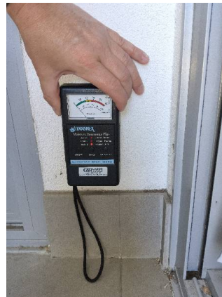
Fiore Apartments – Unit 5 Balcony: Control moisture reading 0 percent.
