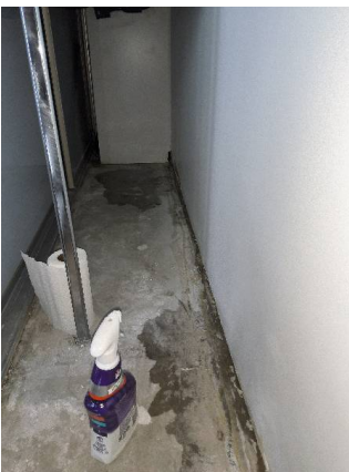
Fiore Apartments - Bedroom #1: View of the built in robe with visible standing water.
