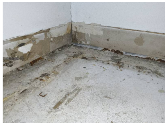
Fiore Apartments – Bedroom 2: Close up view of external corner of robe with visible rust to steel studwork.
