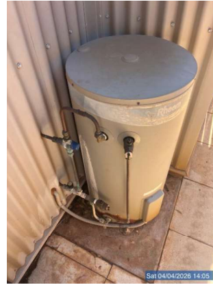
REAR: Hot Water System (photo 1 of 1)
